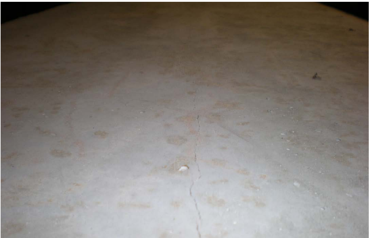
Figure 1-3 Observed Longitudinal Cracking
