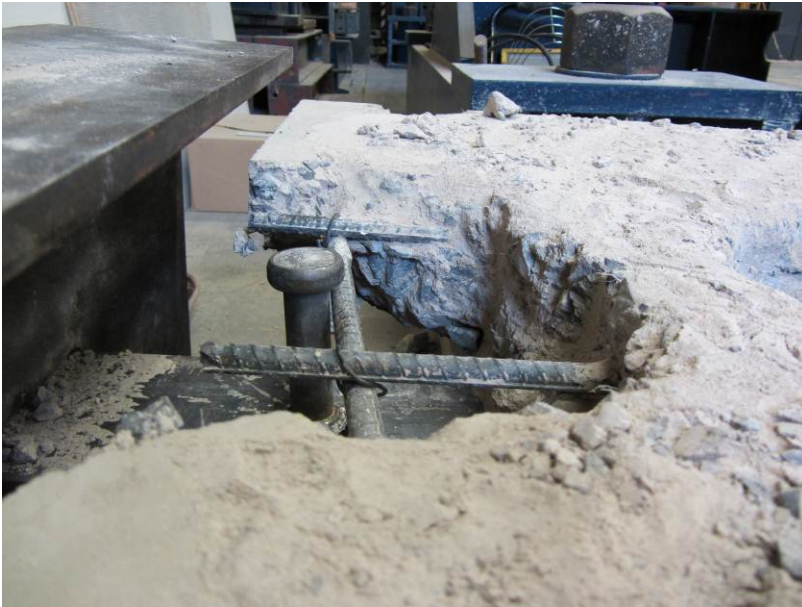
Figure 5-5 End Stud with Concrete Removed
