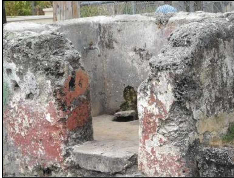
Figure 4-1: A traditional stand pipe where Barbadians used to gather with buckets to supply their homes with water (BWA, 2012).
