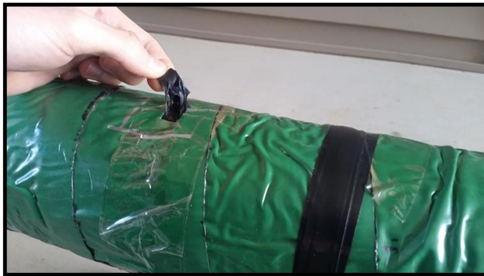
Figure 58: The tar was very sticky and viscoelastic. Notice the air bubbles under the wrap, indicating that the coupling between the tar wrap and the pipe may be highly variable. Adhesion between the tar and pipe should attenuate SH waves due to energy leakage.
