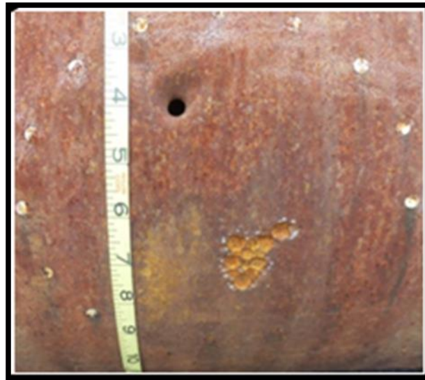
Figure 47: Close-up view of the hole and the simulated pitting corrosion. These two defects are a mere 3" apart.
