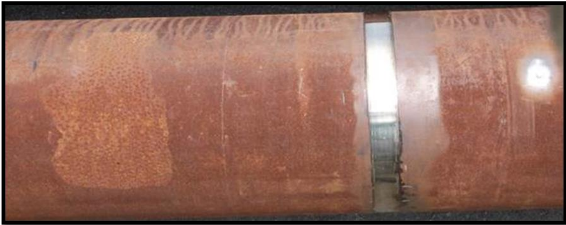
Figure 54: 16” diameter pipe with large simulated pitting corrosion patch, visible to the left of the FeCo strip. The corrosion patch was made by first grinding down the surface to thin the pipe wall, and then drilling many small spherical pits. The grinding reduced the wall thickness by a few millimeters, and each pit is another few millimeters deep.
