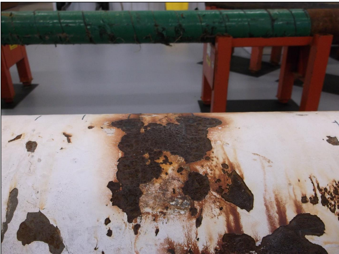
Figure 4: An example of localized pitting due to external corrosion on a steel pipe.
