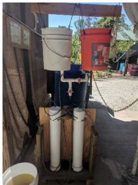
Figure 17. Large scale Moringa filters constructed by ECHO Appropriate Technology
