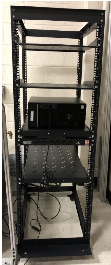
Figure 8. Server rack behind testbed to house computer and eventually all circuitry
