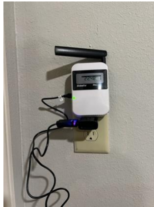
Figure 3.7 The GlobalSat Air Quality Monitoring Sensor
